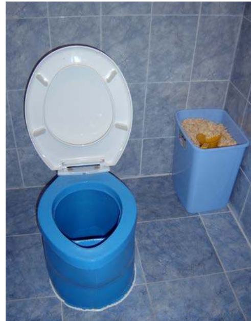
Interior of an Ecosan toilet (UDDT) cabin, constructed inside of a house in Bulgaria. Photo: Earth Forever
