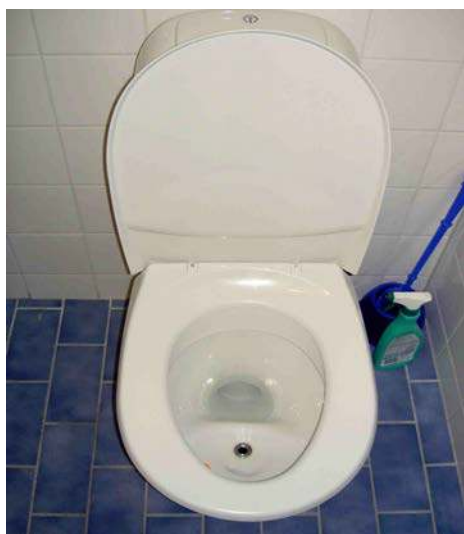
Urine diverting toilet with water flush
