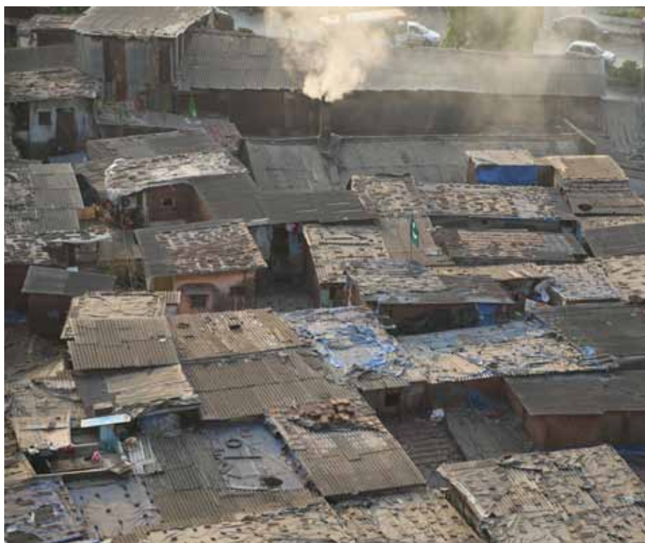
Asbestos containing roofing materials, © ROCA/GAAA
