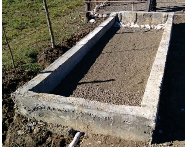
Figure 7: A horizontal greywater filter in the project region, between construction and planting.
