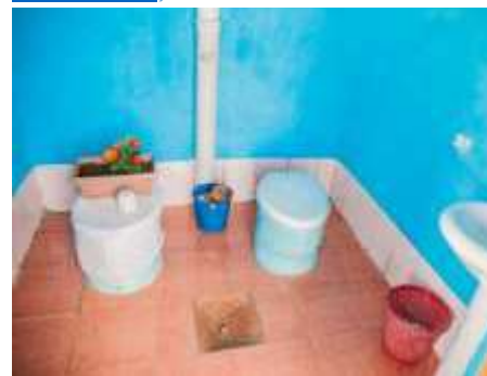
Interior of a UDDT cabin (source: WECF)
