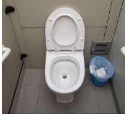
JETS 50M vacuum toilet inside Lau Fau Shan Roundabout Public Toilet (source: Wrightbus, 2011 )
