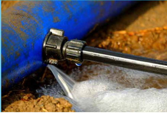
Corrosion can cause severe leakages in the distribution system (source: Holger Schué)
