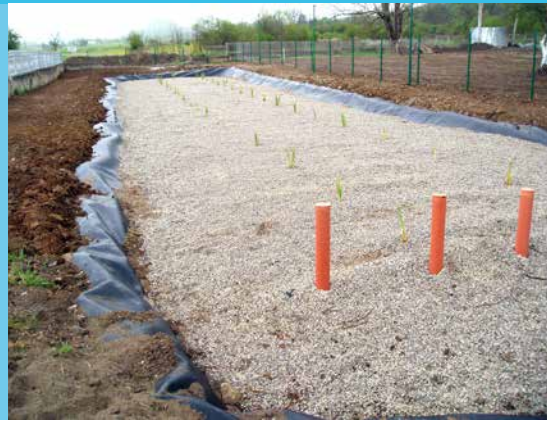
Constructed wetland used for decentralised treatment of wastewater (source: WECF)
