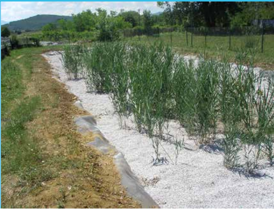
Constructed wetland, Bulgaria (source: WECF)
